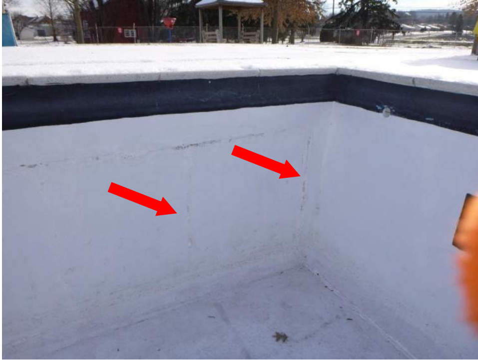
Photo #9 – Cracks in pool walls in multiple locations
