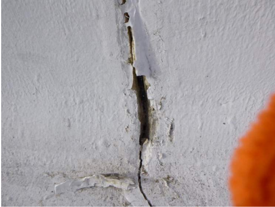
Photo #7 – Crack in pool wall and slab, deteriorated sealant
