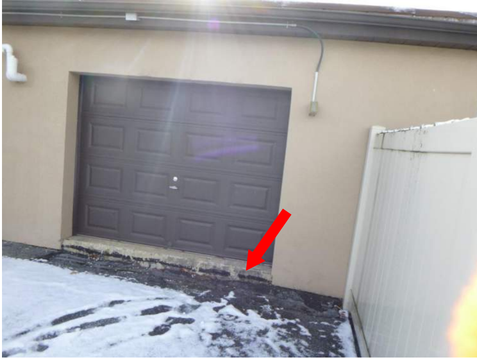
Photo #3 – Settled pavement on left side, cracks and depressions noted
