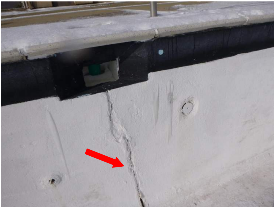
Photo #8 – Cracks in pool walls in multiple locations
