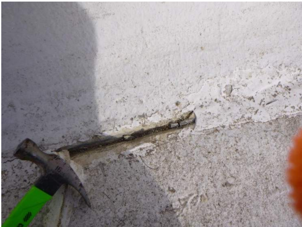
Photo #6 – Deteriorated sealant and separation between dividing wall and pool slab
